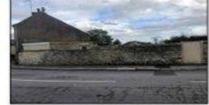
Corner Cottage, existing flat roofed extension and boundary wall viewed from the west
